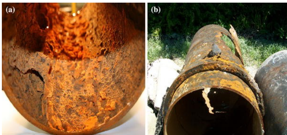
Figure 1. Inner pipeline corrosion (Choi, et al., 2015)
